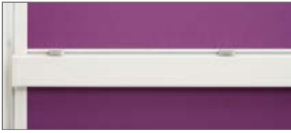
External cable management
